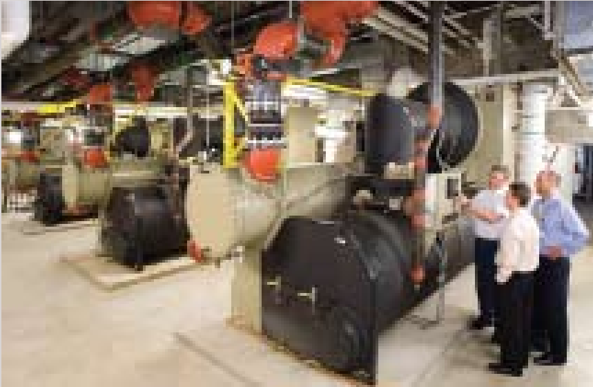
As part of Gundersen Lutheran's retrocommissioning process, changes were made to the chiller's system programs to optimize cooling tower fan utilization with the chiller compressor.
