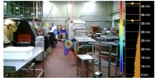
Above: Sonic imaging readout detects previously hard-to-access air leaks through SugarCreek's award-winning project.
